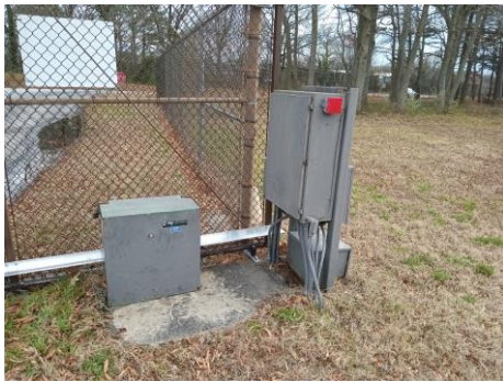
SLIDE DRIVER AND JUNCTION BOX
