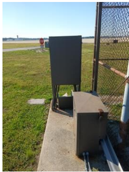
SLIDE DRIVER AND JUNCTION BOX
