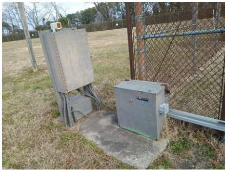
SLIDE DRIVER AND JUNCTION BOX
