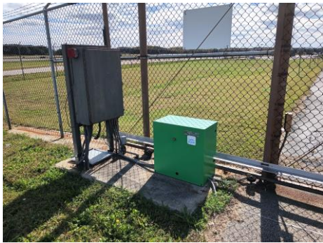
SLIDE DRIVER AND JUNCTION BOX
