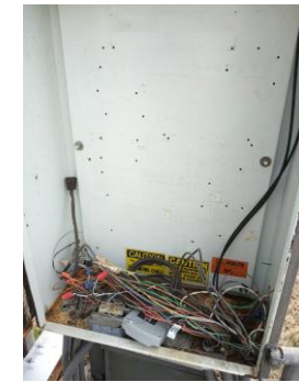
JUNCTION BOX OPEN
