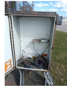
JUNCTION BOX OPEN
