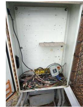
JUNCTION BOX OPEN
