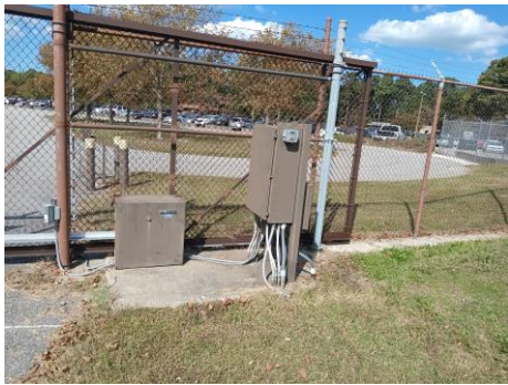
SLIDE DRIVER AND JUNCTION BOX
