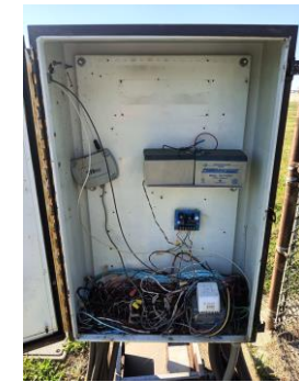
JUNCTION BOX OPEN
