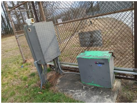
SLIDE DRIVER AND JUNCTION BOX
