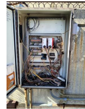
JUNCTION BOX OPEN
