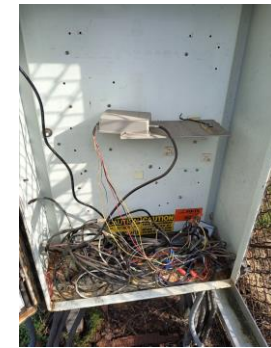
JUNCTION BOX OPEN
