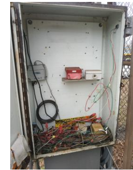
JUNCTION BOX OPEN
