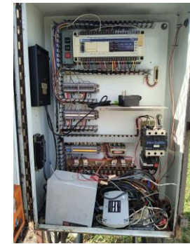
JUNCTION BOX OPEN
