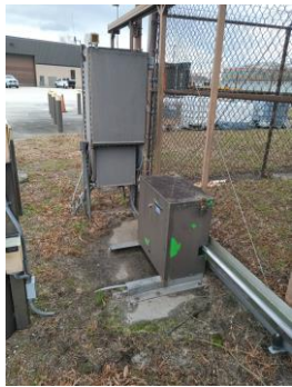
SLIDE DRIVER AND JUNCTION BOX
