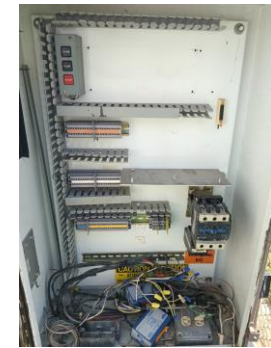
JUNCTION BOX OPEN
